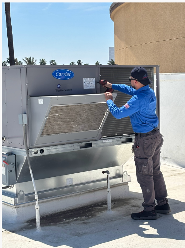
Mechanical Air technicians servicing an HVAC unit to ensure safe, efficient heating and cooling for Central Valley customers.
