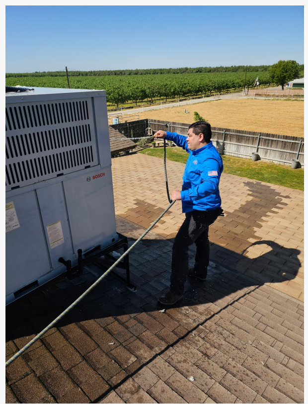
Mechanical Air technician cleaning an HVAC unit to improve efficiency and ensure reliable performance.
