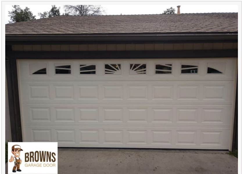
Recently Completed Garage Door Installation by Brown's Garage Door – Quality You Can Rely On
