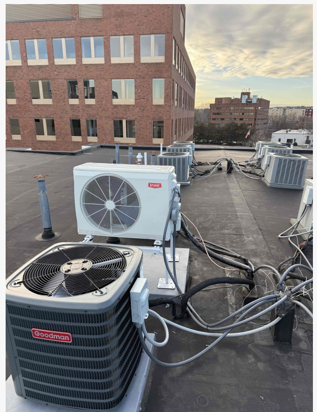
Bryant Heat Pump installed in Boston Metrowest by Endless Energy
