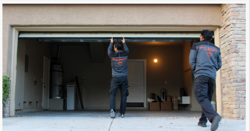
An Open Sesame technician performs an emergency garage spring replacement for a home in the Summerlin area.
