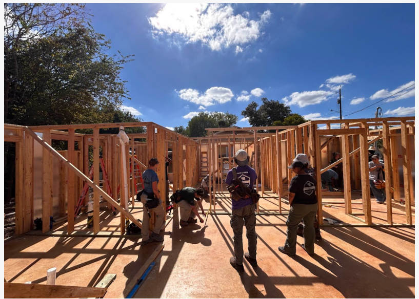
YouthBuild members in construction training build homes while preparing for careers in the skilled trades.
