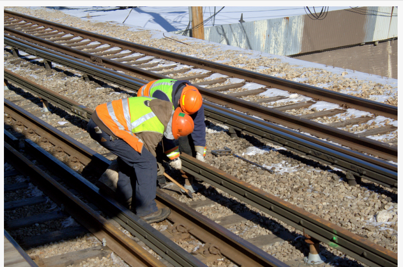
Transit Workers use the TESCO Third Rail Voltage Detector
