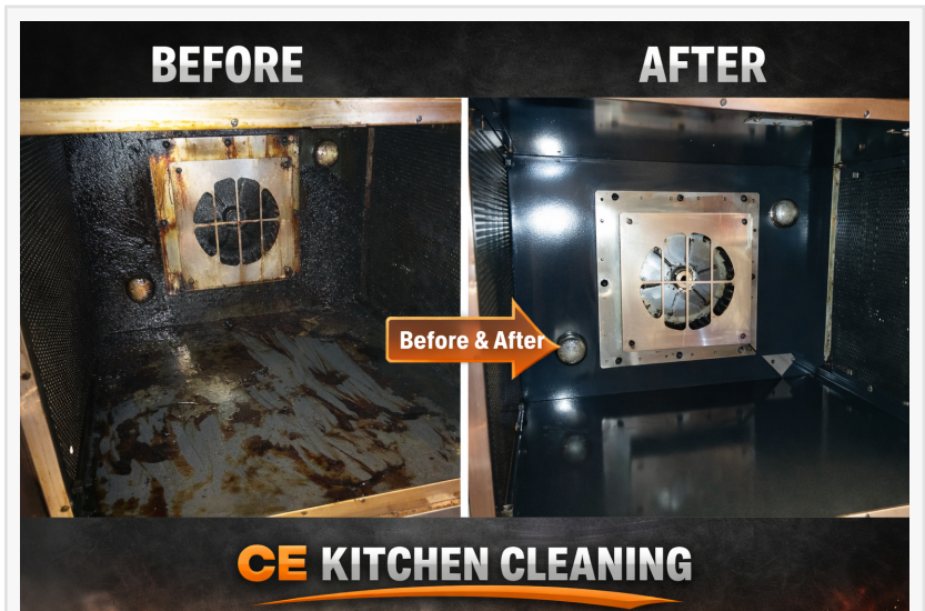
From Heavy Grease Buildup to Sanitized Surfaces: A Professional Kitchen Deep Clean
