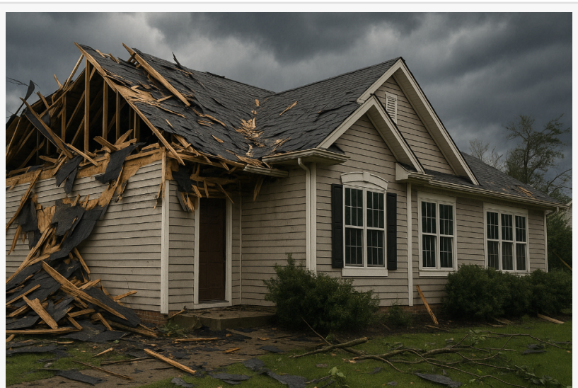
WRC Assists When Storm Damage Occurs
