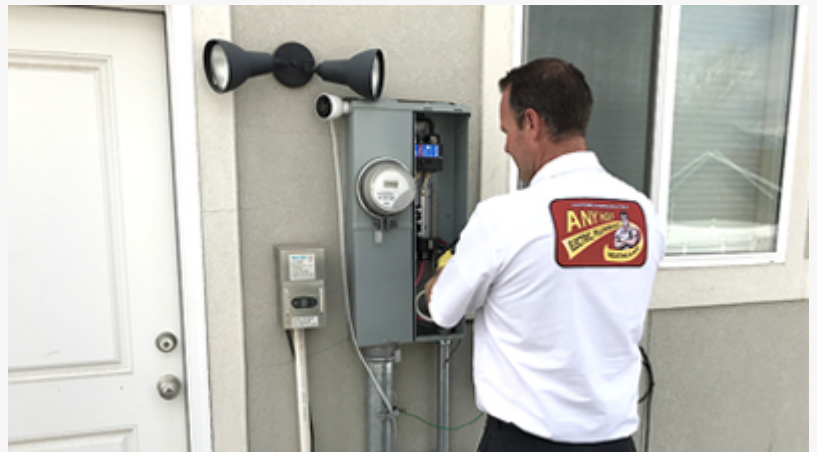
An Any Hour technician examining an electric panel.
