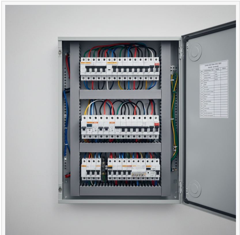
Neatly organized electrical breaker panel with labeled circuits.
