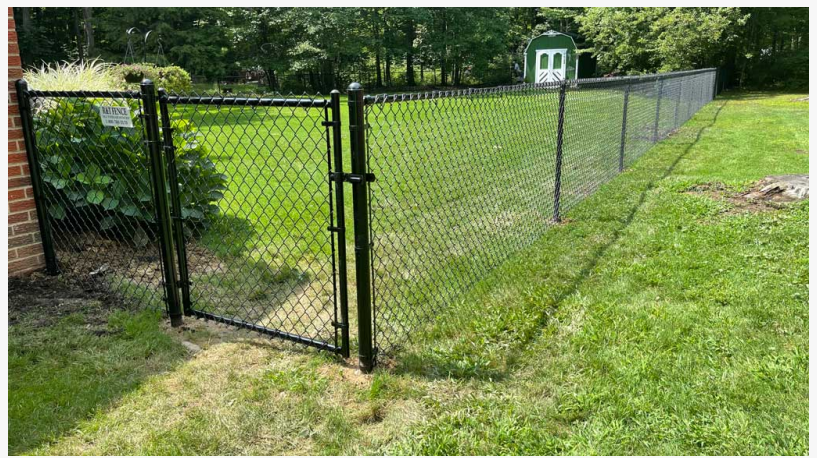
Black chain link fence installed along a residential backyard property line to provide security while maintaining visibility.
