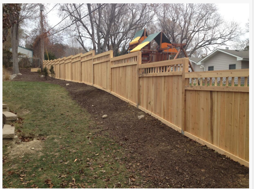
Custom wood privacy fence installed on a sloped residential property, designed to enhance privacy and complement the surrounding landscape.
