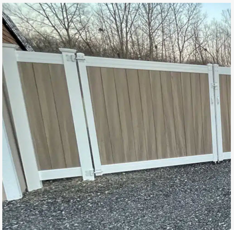
Vinyl privacy fence installed around a residential yard, offering a low-maintenance solution for privacy and property separation.
