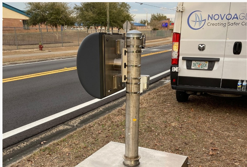
NovaGlobal School Zone Speed Enforcement Camera in Crestview, Florida
