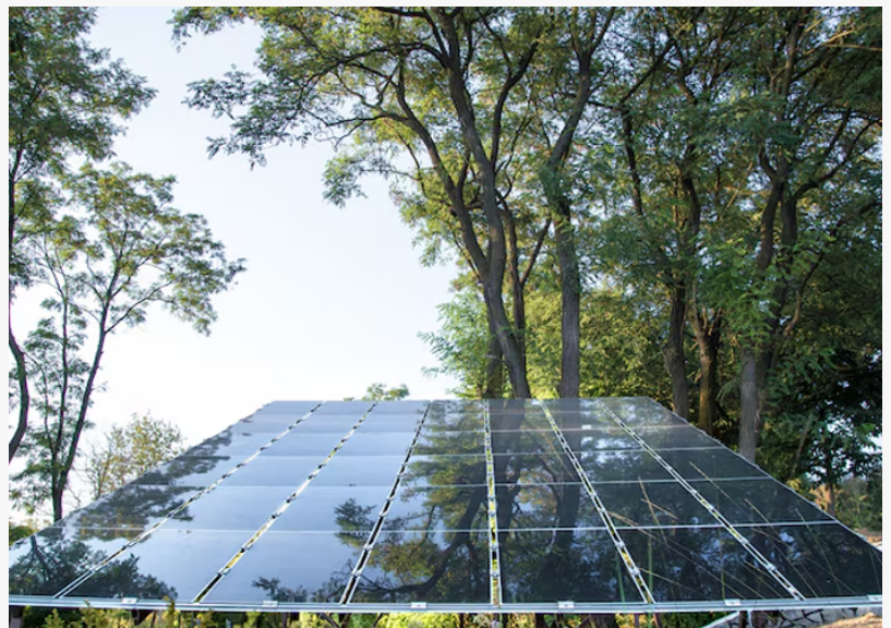
residential solar panel system pitkin
