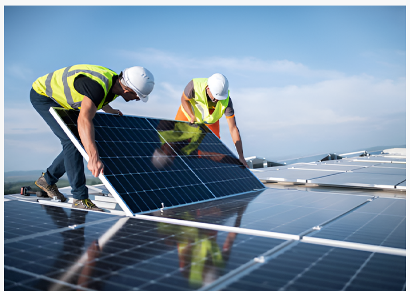
residential solar panels Garfield
