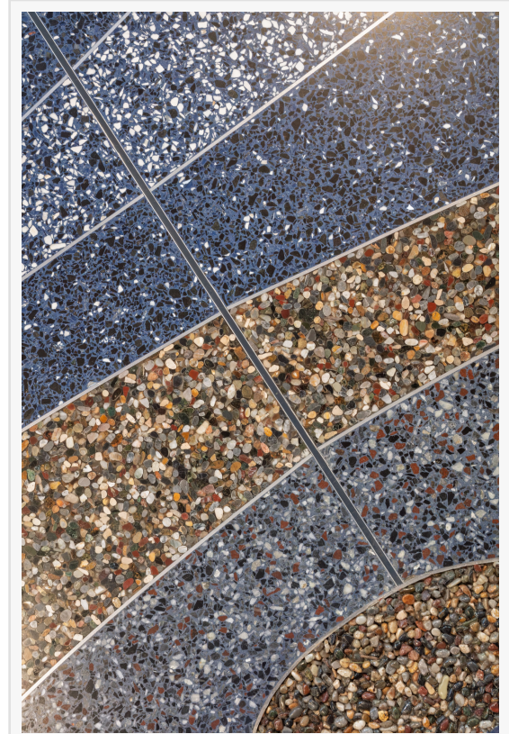
Kankakee Welcome Center's terrazzo in shades of blue, with river rock and a rustic finish represents Indiana's waterways.
