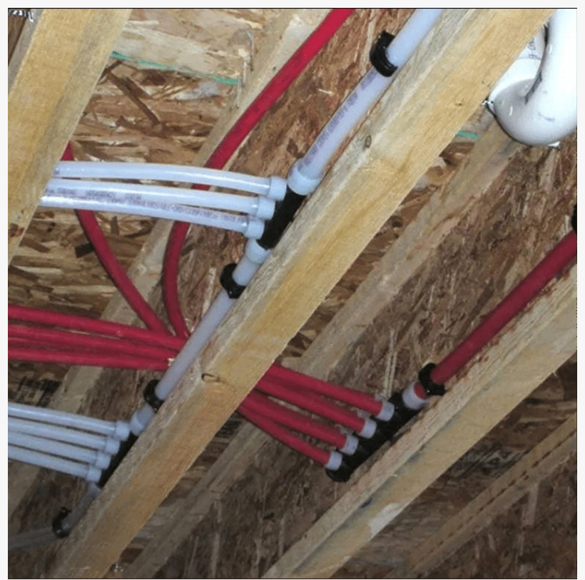
New Uponor PEX-A water lines installed during a whole-house repiping project in Pasadena, Texas, replacing aging galvanized plumbing to improve water pressure and prevent future leaks.
