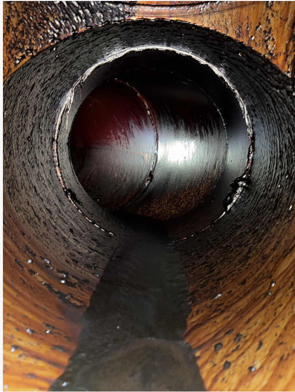
A dirty exhaust duct that is about to be cleaned by a Filta Kleen technician
