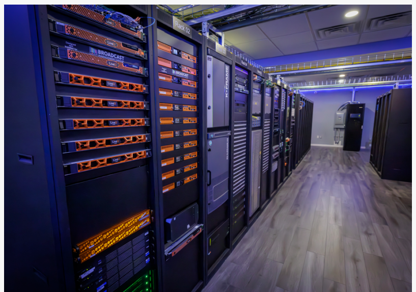
Broadcast Media Asset Management Data Center
