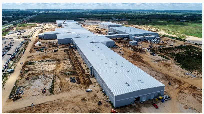
Aerial view of Navistar's 1,000,024-square-foot manufacturing facility in San Antonio, Texas, supported by more than 6,000 tons of structural steel supplied by Allied Steel Buildings.
