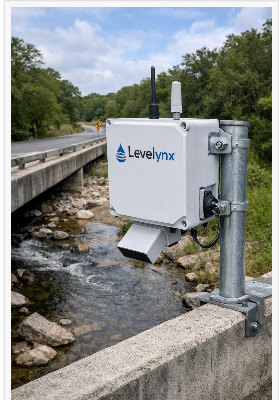
Levelynx radar-based flood monitoring system installed above a creek crossing in Central Texas.
