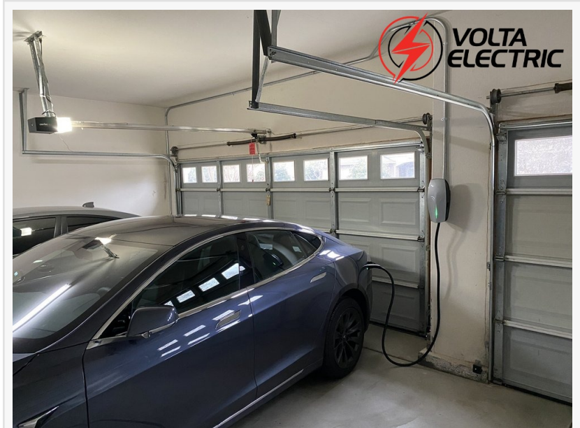
A car being charged from an EV charger in Santa Monica installed by Volta Electric
