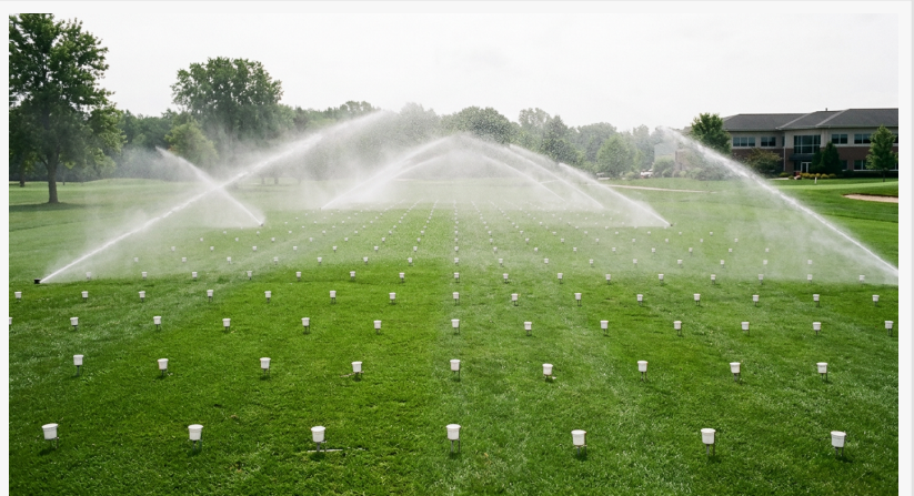
Catch-can audit in progress on a commercial property lawn, measuring distribution uniformity across the irrigation zone.
