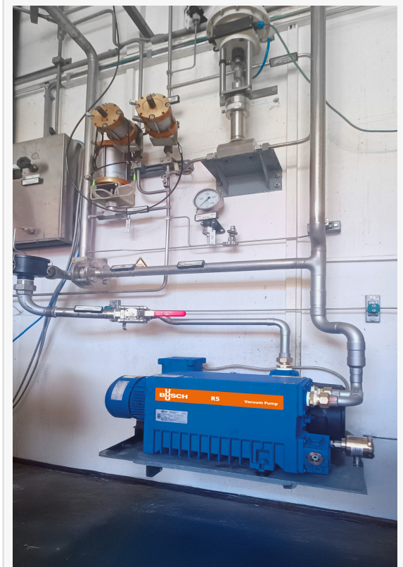
Hydrogen version of the R5 ATEX installed at Air Liquide Austria GmbH. Source: Busch Group.
