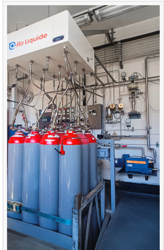
Bottling plant for special gasses from Air Liquide Austria GmbH. Source: Busch Group.
