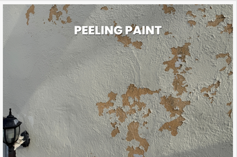
Peeling paint over stucco
