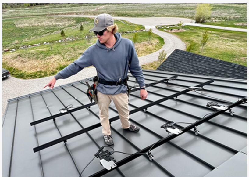
commercial solar power installation Garfield
