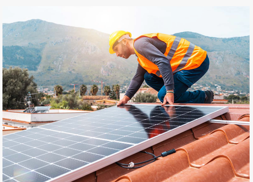
commercial solar panel installation Garfield
