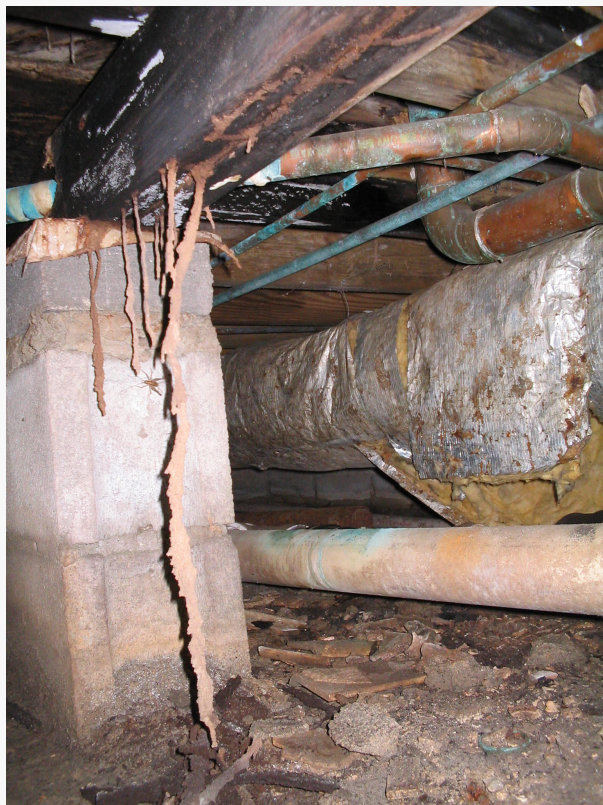
Termite Tubes Under Home
