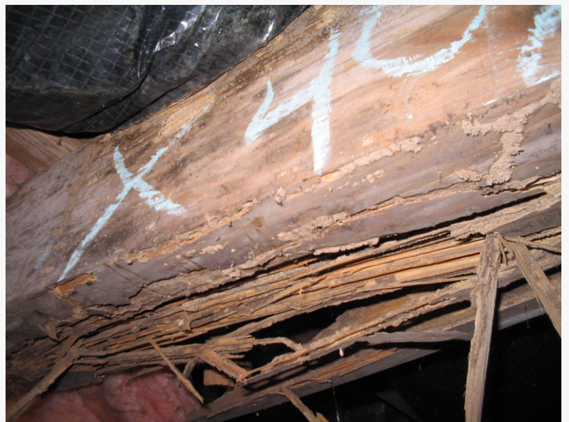
Termite Damage in Virginia Beach
