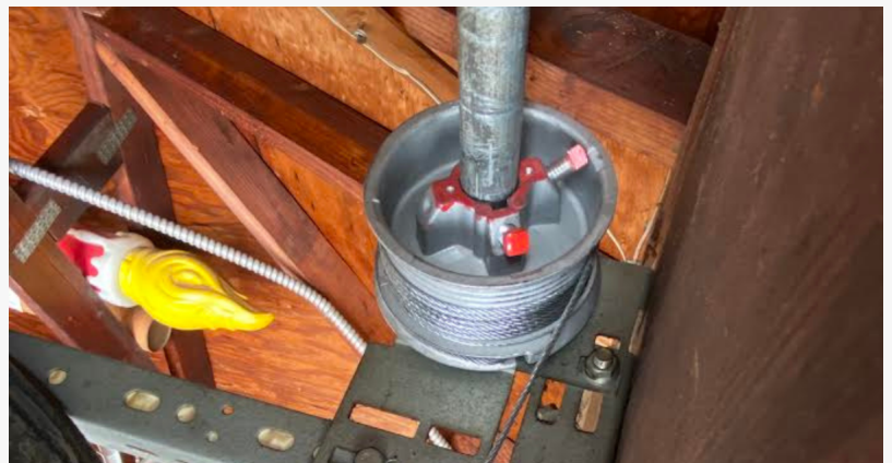
A certified technician safely replacing a broken, heavy-duty torsion spring on a residential garage door.
