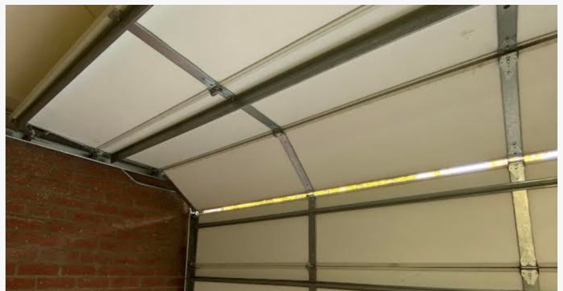
An expert installing a new, quiet smart garage door opener system on the ceiling of a garage.
