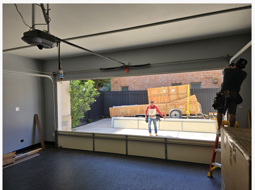
Upgrading a noisy garage door in Oak Ridge North with ultra-quiet, sealed nylon rollers for smooth, silent operation.
