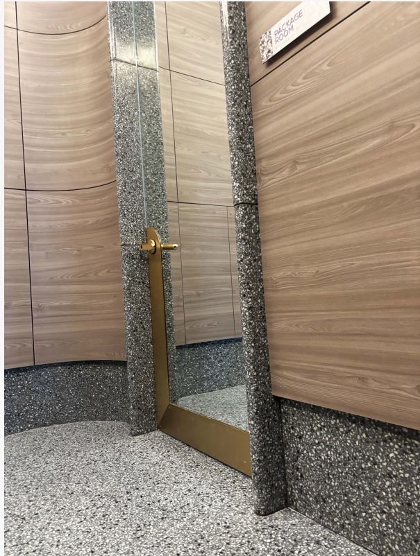
Terrazzo portals with concealed door frames and tight joints showcase the project's exacting coordination across trades.
