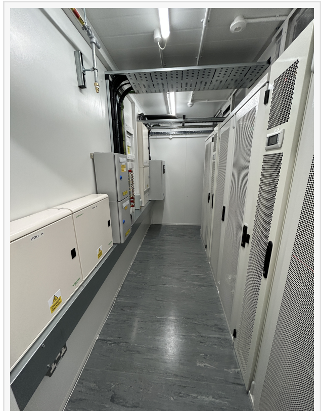
Interior of one of the new data centres
