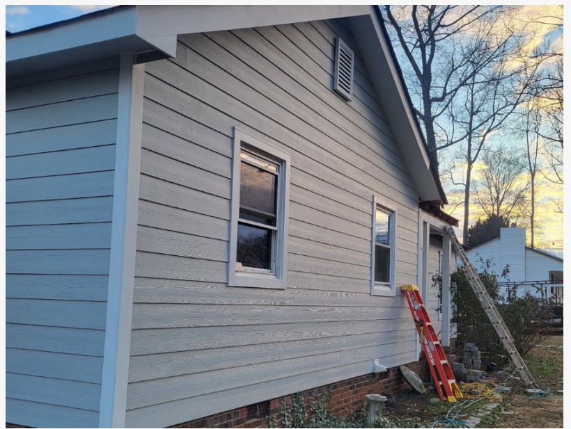
James Hardie fiber cement siding with woodgrain texture installed by Hatch Homes
