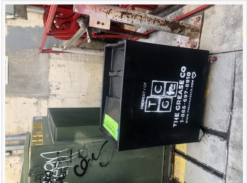
Grease trap installed in a commercial kitchen for separating FOGS from wastewater
