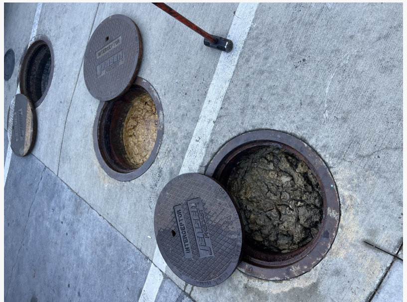
Open grease interceptor undergoing routine cleaning at a commercial facility
