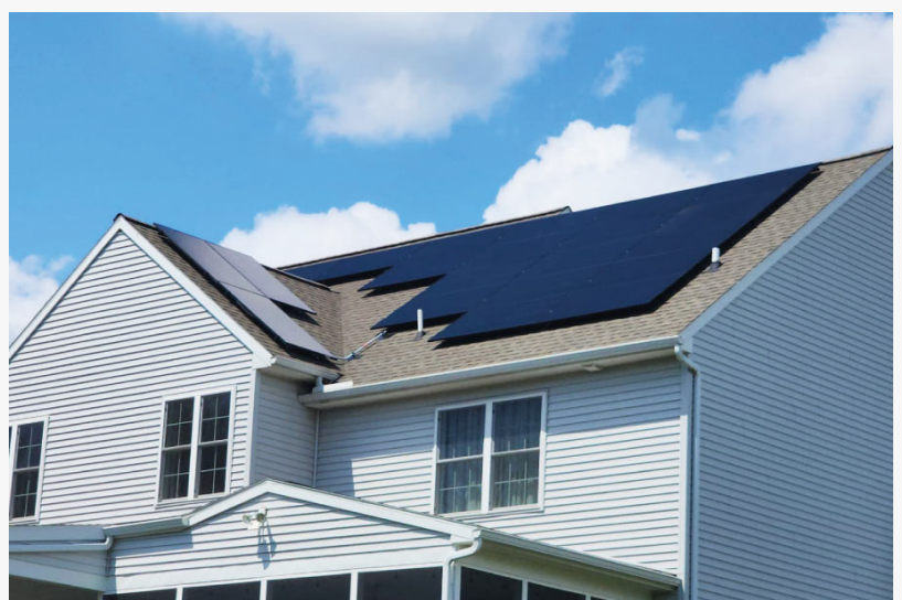
Deep blue solar panels stand out in sharp relief against the light gray of the house siding and the soft whites of the cumulus clouds.
