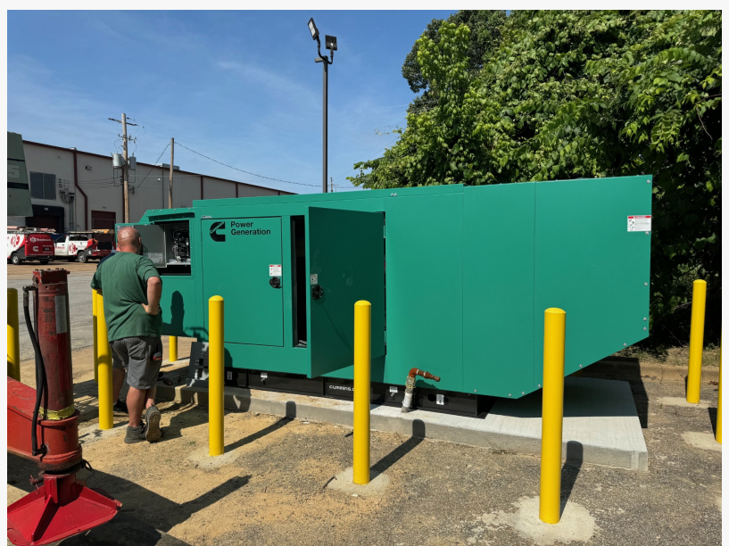
View of Cummins generator installation at UKG-Memphis
