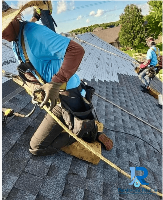
Rainforcing Roofing Experts Ensuring Code Compliance and Fall Safety During Central Illinois Shingle Installation
