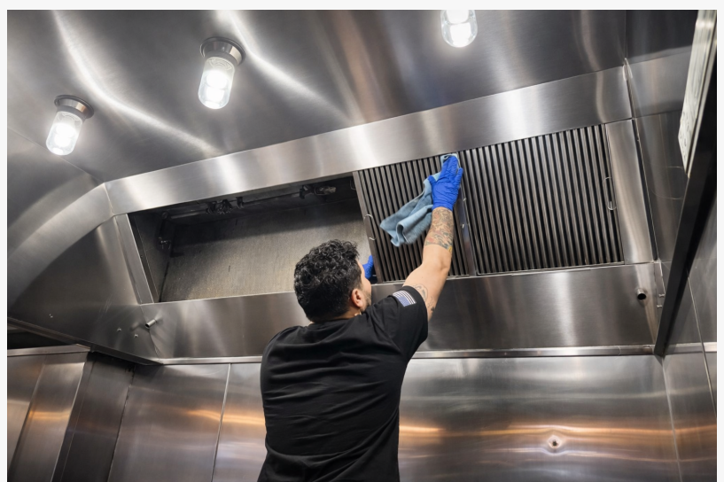
Technician performing deep cleaning of a commercial kitchen exhaust system to remove hidden grease and reduce fire risk
