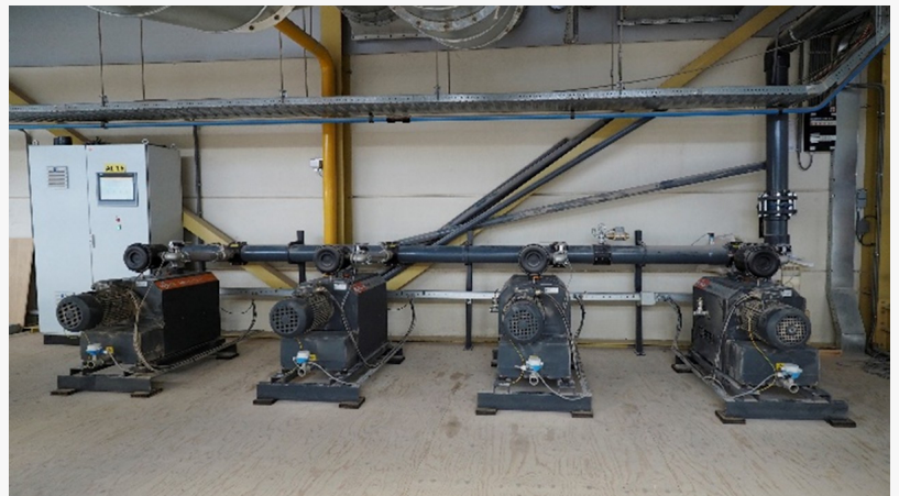
Four MINK vacuum pumps are connected to seven CNC routers. Photo: Busch Vacuum Solutions.
