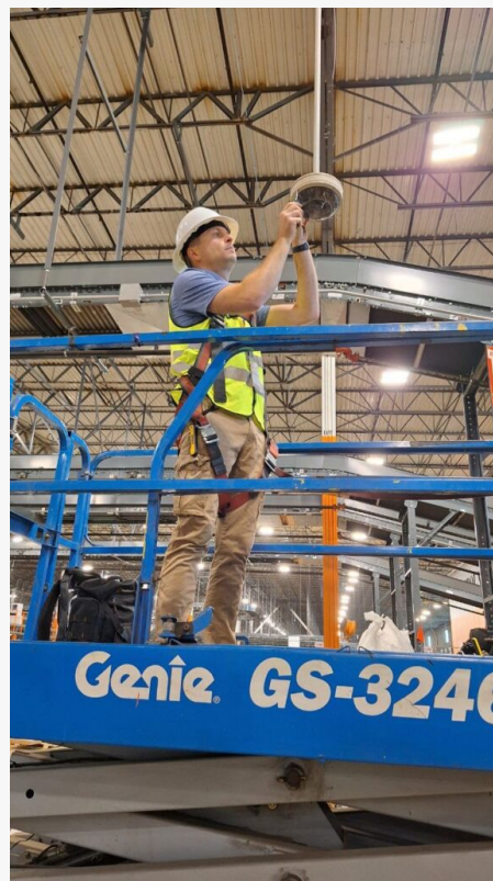
Communication Installation Services
