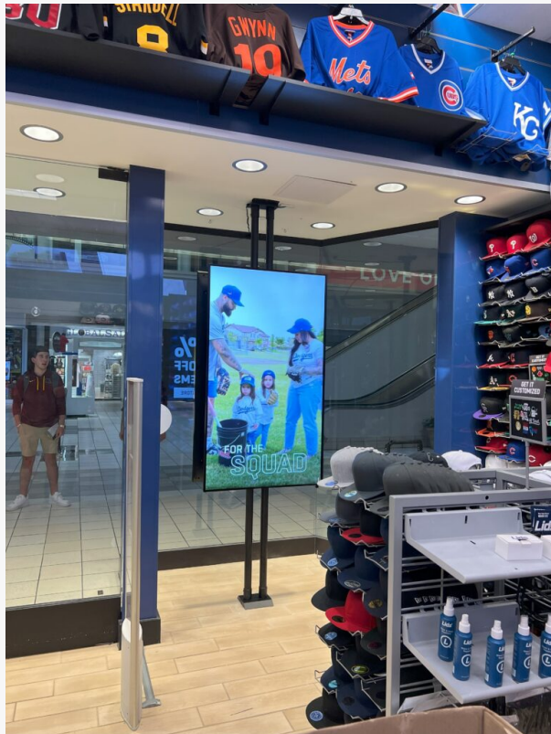
Telecommunication and wiring services
