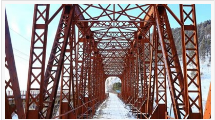
Corrosion on Bridge
