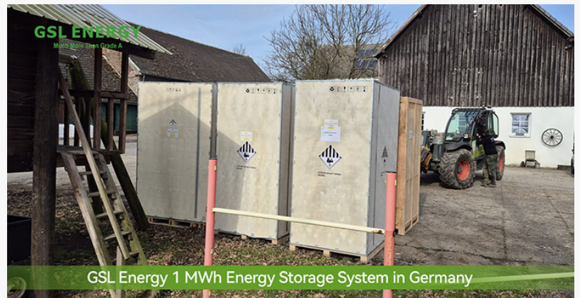
GSL Energy 1 MWh Energy Storage System in Germany
