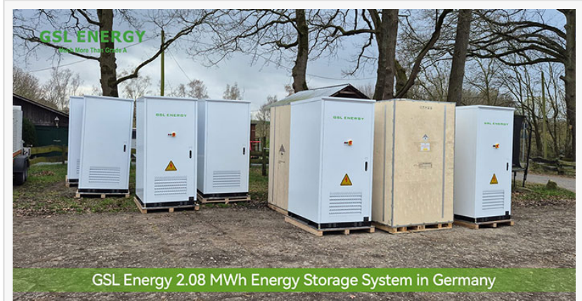
GSL Energy 2.08 MWh Energy Storage System in Germany
