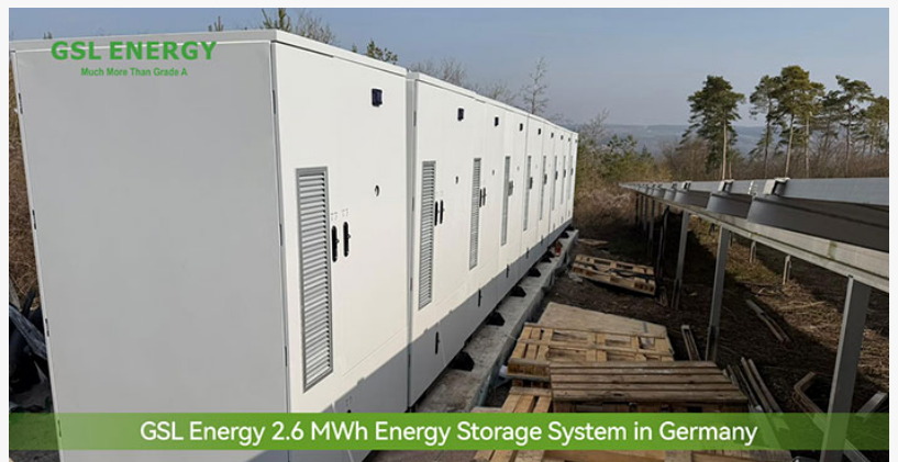
GSL Energy 2.6 MWh Energy Storage System in Germany
