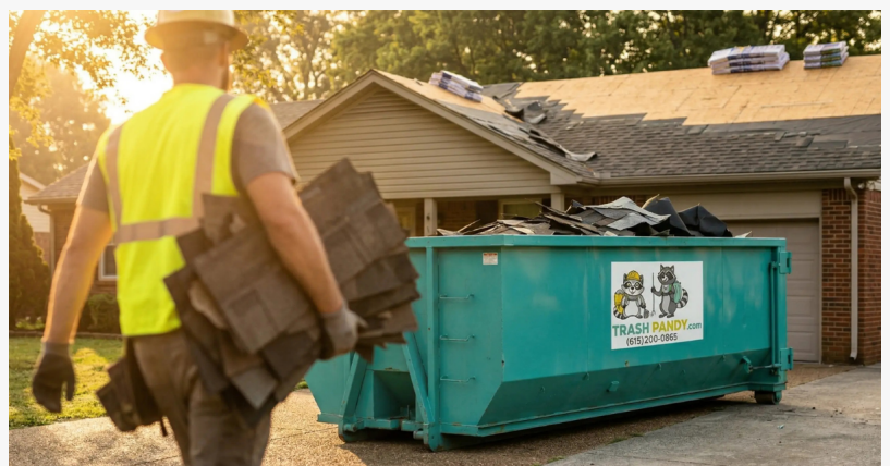
A roofer loads old shingles into a branded Trash Pandy dumpster during a residential roof tear-off near Murfreesboro, Tennessee.
