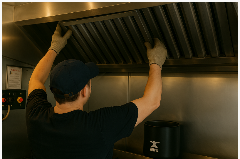
A Done Right worker installing a commercial kitchen hood at a Miami restaurant
