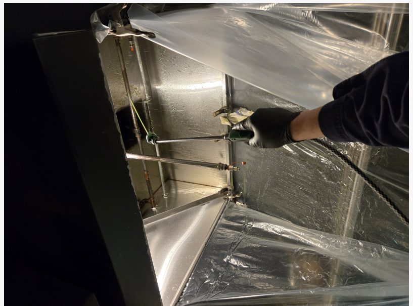
A Done Right hood cleaning specialist cleaning a commercial kitchen's canopy at a local restaurant
