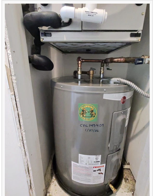
38 gallon lowboy water heater installation completed by Plumbing Detectives LLC serving Venice and Sarasota County Florida.
