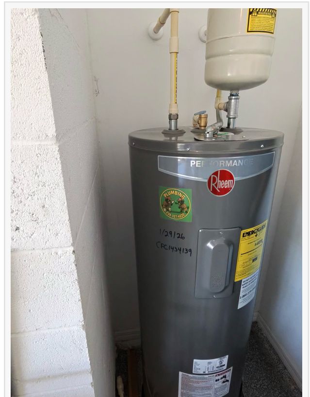
Water heater installation completed by Plumbing Detectives LLC in the Venice, Florida service area.
