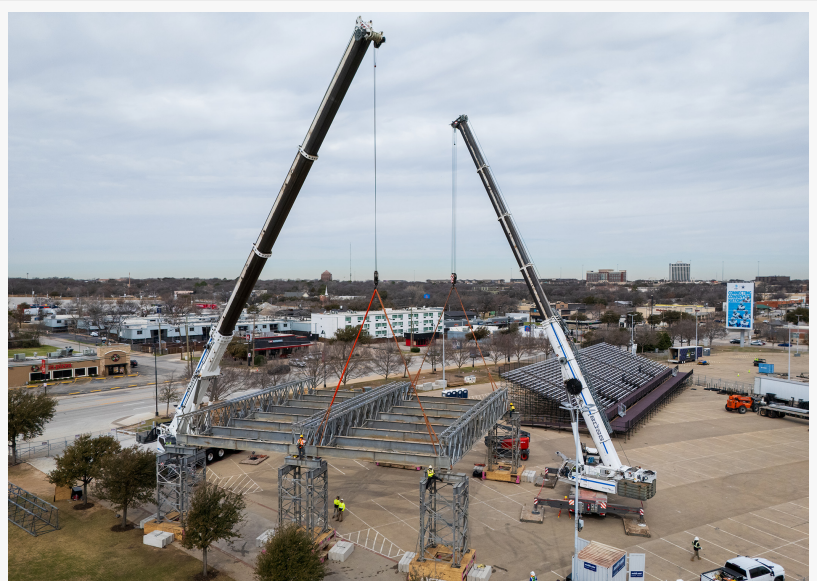
BOSS Crane uses a GMK7550 all-terrain crane on one end and a GMK6300L to tandem lift the Horseshoe Club section into place.
