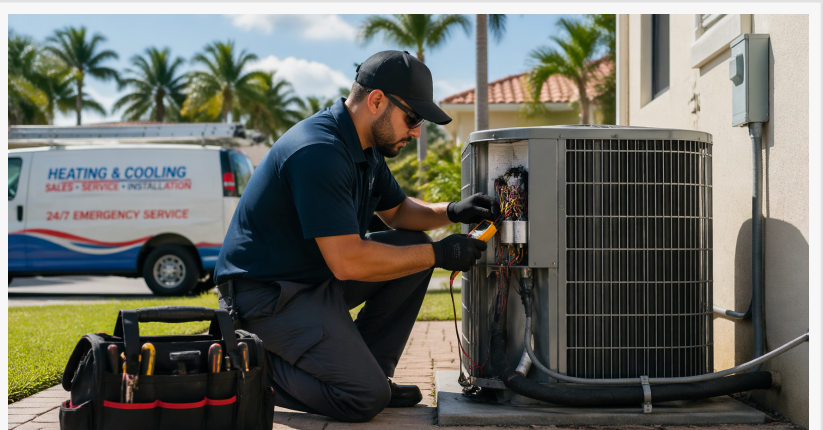
HVAC technician working on an outdoor air conditioning unit at a residential property in Greater Miami ahead of peak summer demand.
