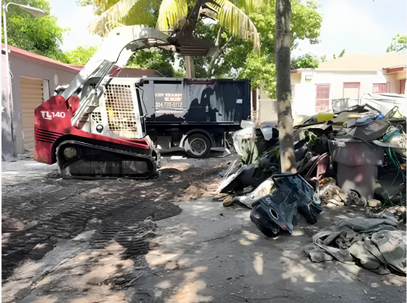
Land clearing and debris removal by XS Trash in Broward County using bobcat equipment for large property cleanouts and construction cleanup projects
