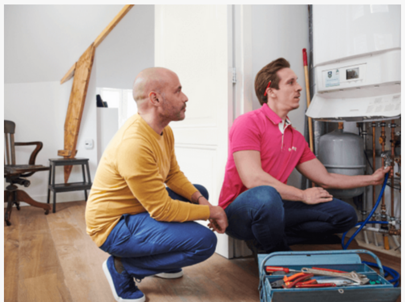
Essent specialists maintain boiler
