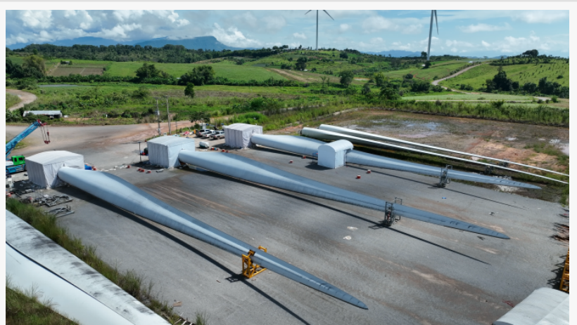
CEWA Plus will conduct blade root manufacturing across Asia using We4Ce's Re-FIT method and CNC Onsite's mobile machines
