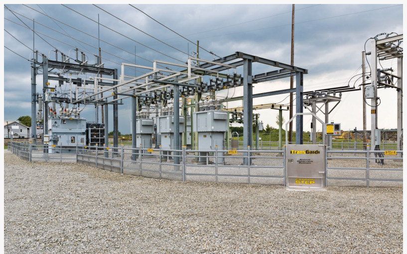
TransGard has announced the installation of its 5,000th substation fence
