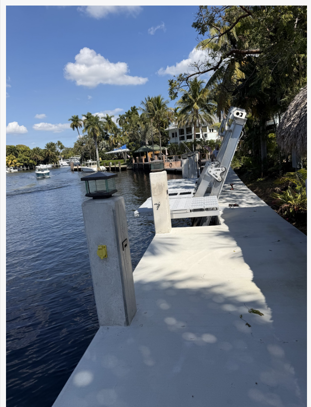
A recently completed seawall installation in Broward County by South Florida Seawall, built to meet the 5.0 feet NAVD88 minimum elevation required under Fort Lauderdale's tidal flood barrier ordinance.
