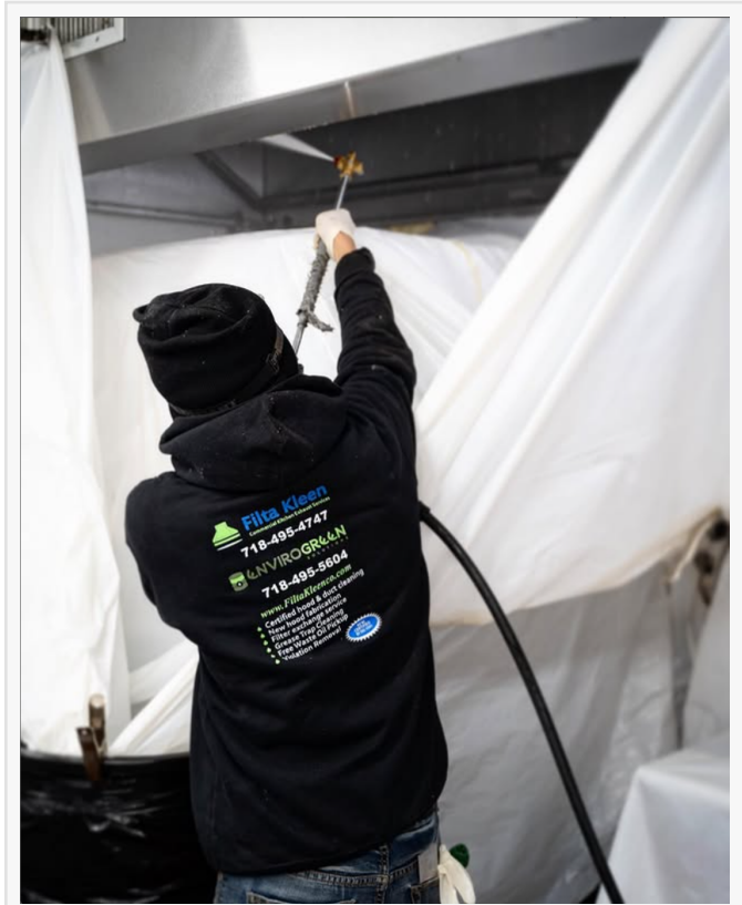
A Filta Kleen Hood Cleaning Specialist Cleaning a Commercial Air-Duct.
