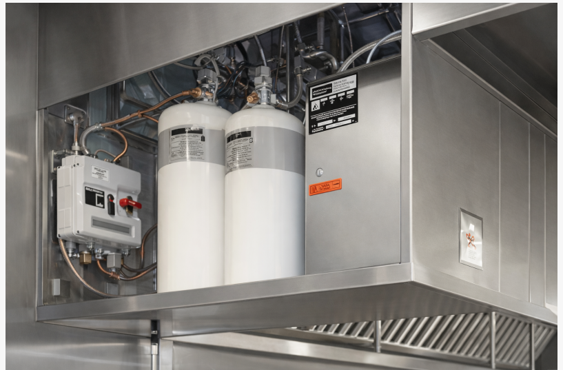
A fire suppression installed on a restaurant hood at a local NYC eatery
