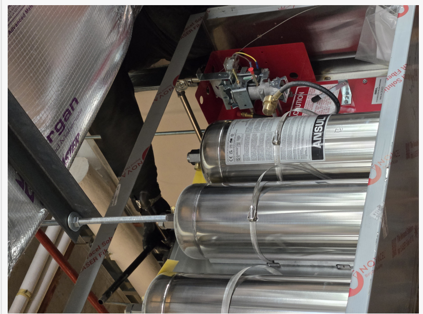
A Ansul Fire Suppression System installed in a restaurant that Done Right Hood and Fire Safety Services Located in South Florida
