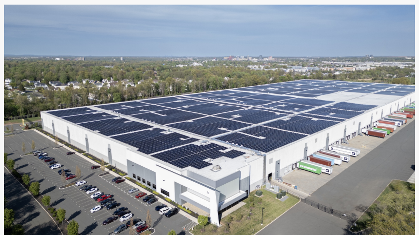
NJ's largest ever rooftop community solar installation.
